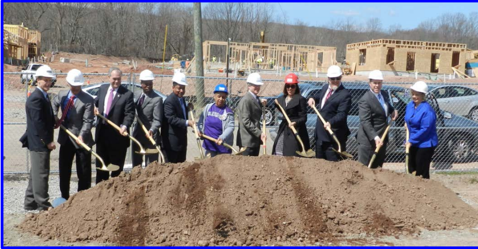
Rockview Terrace (groundbreaking) 300 Wilmot Road ■ New Haven 77 units of family / supportive housing
